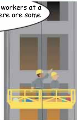
Well-built suspended scaffolds, with steel cables in good condition and well fixed.
